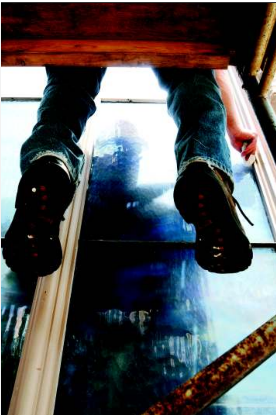
Jerome Durr works on glazing the protective layer of clear glass on the outside of the church as he sits on the scaffolding facing the window. Because of the help from his studio assistant Brad Sliter and James Dunster, who replaces the wooden frame components and the sill plate on the exterior, Durr was able to finish ahead of schedule.
