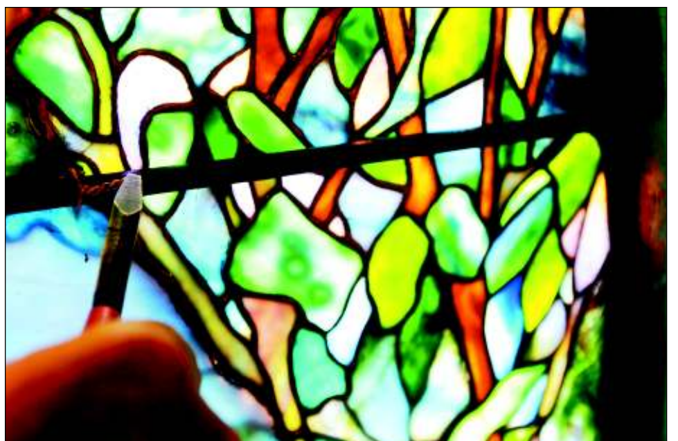
Pliers are used to tighten the metal ties that are soldered to the window. The ties wrap around the metal bars that run through the wooden window frame to hold the panes in place.
